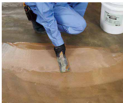
After applying Dynamic load resistant floor Primer, apply using a plastering brush, rubbing into subfloor.
