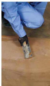
(5) After Dynamic load resistant floor Primer dries, apply Dynamic load resistant floor Hardener
